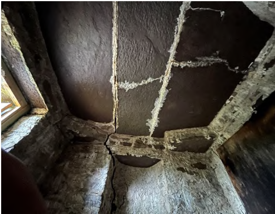
Stone slabs forming ceiling (note lateral cracks marked by lime deposits)
